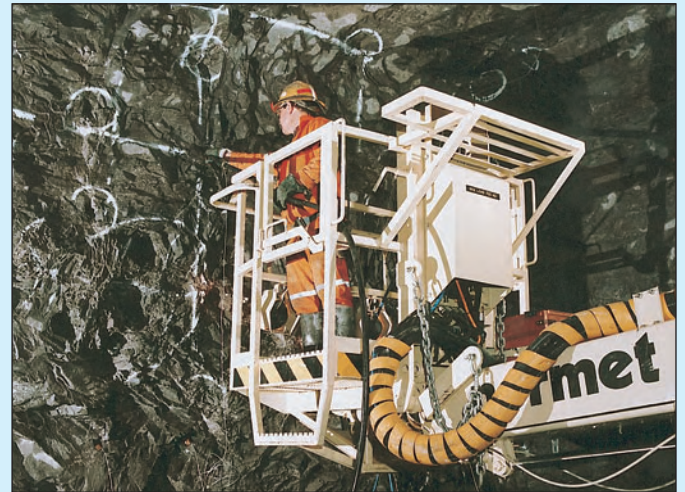
Preparing for a blast at the underground Navan Zn-Pb deposit. (Courtesy : Tara Mines Ltd.).
